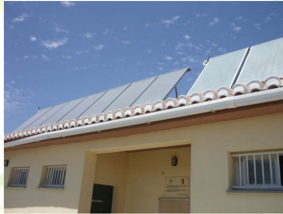
Figure 8 Solar collectors for sports facility in Padul
